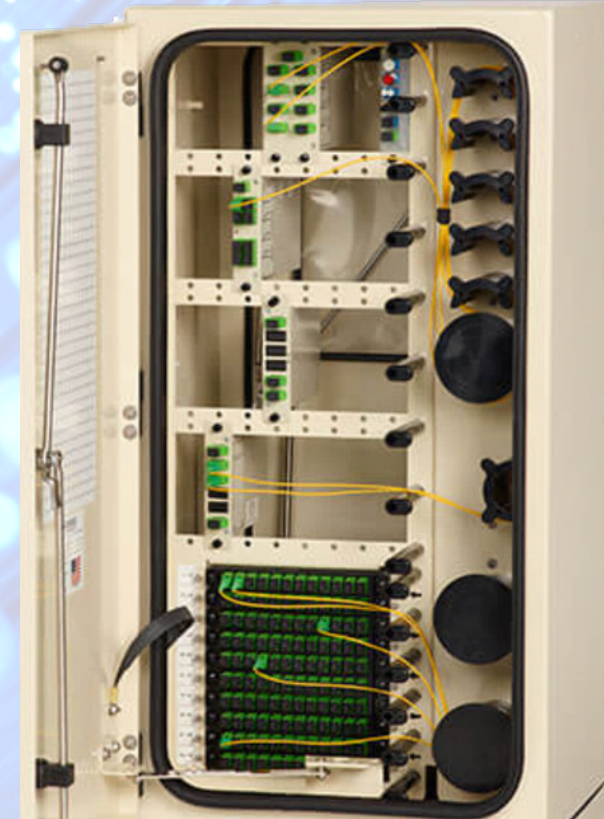
Fiber Distribution Hub
